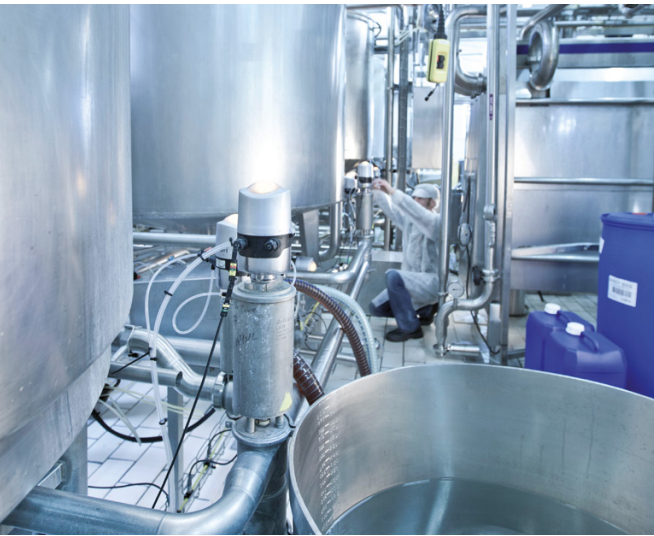
Media preparation tanks
